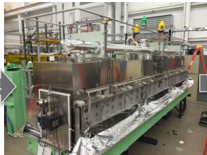
Completed cryogenic circuit
